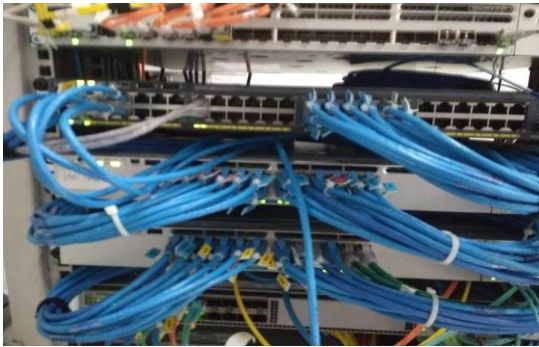
Gambar 15. Server - Core Switch Distribution
