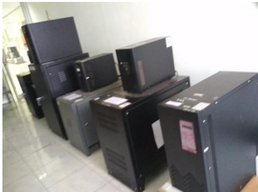
Gambar 10. UPS (Uninterruptible Power Supply)
