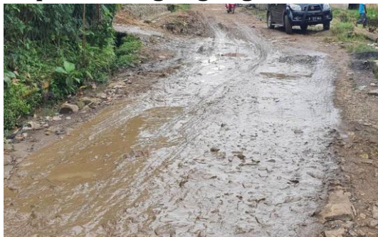
Figure 2. Damaged Road Infrastructure in One District in Dapil 2 Pandeglang Region
